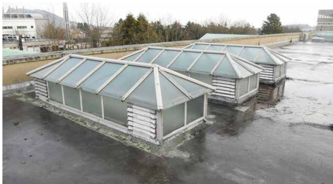
BEFORE: Single skin glass units allowed water ingress and provided poor thermal insulation
